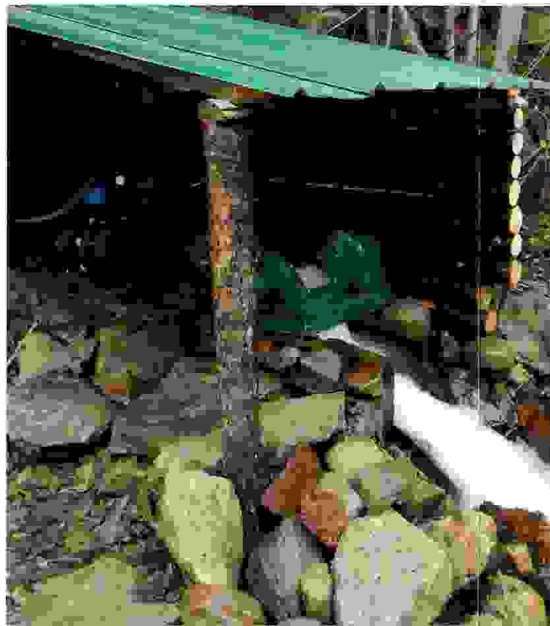
No dam is required, only an upstream diversion through a 6" pipe, which is coupled to the unit.
